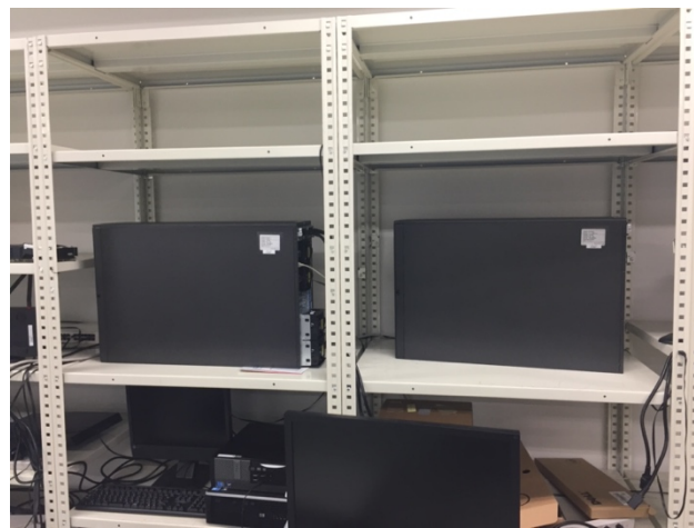
Fig. 2. GPGPU parallel computing servers.
