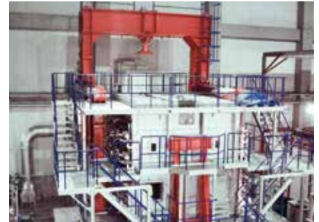
Multiple Full-scale Furnace
